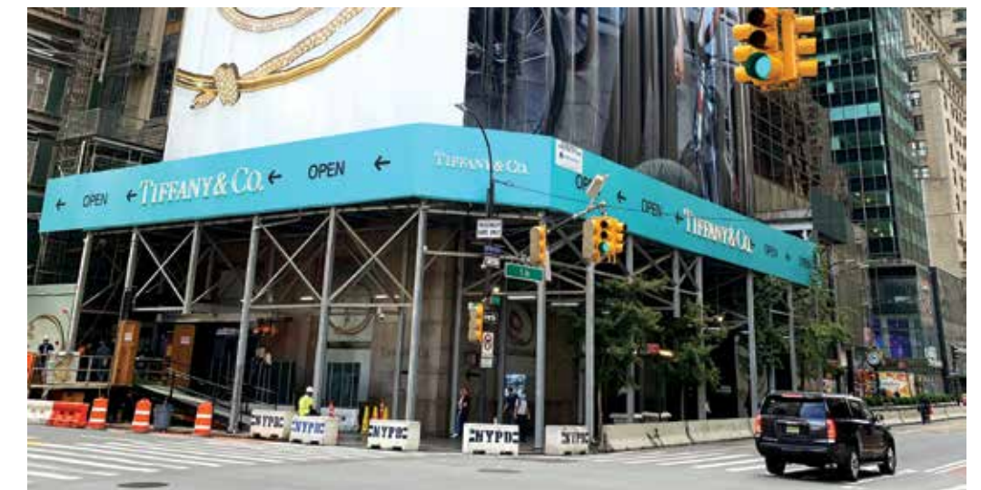
Renovation of Tiffany & Co.’s Manhattan flagship store is expected to finish by end-2022. Source: Paul Zimnisky
